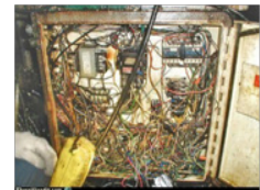
appropriate for the Fig 4.6 : poor wiring
